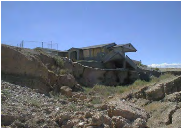
Unstable Slopes along the bluffs south of the Colorado River, west of the Redlands Parkway
